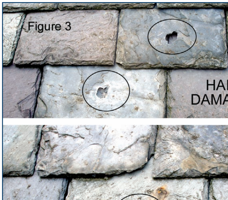
Figure 3 – Hail-perforated slates should simply be removed and replaced. Hail damage rarely justifies replacement of an entire slate roof.
